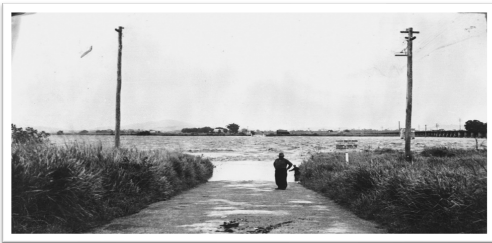
Plate 14.70: Here, the Pioneer (Hospital) Bridge over the Pioneer River has disappeared under floodwaters. The bridge was low, with no railings, so that floodwater would go over the top.
